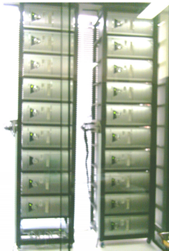
Fig. 3. In the picture it appreciates the physical disposition of the cluster. This is a rack with 19 nodes.
